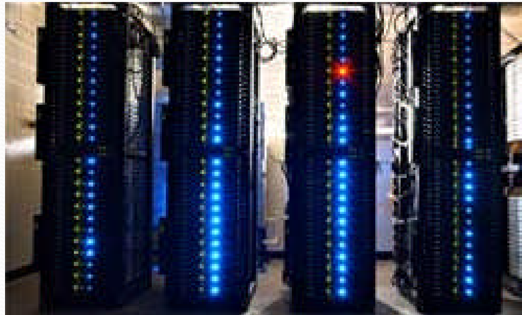
Web server racks
